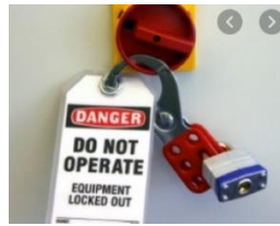
Fig. Error! No text of specified style in document..3 Electrical Lock-out system
