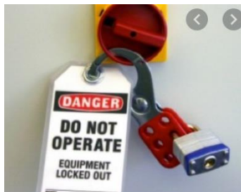
Fig.4. Electrical Lock-out system
