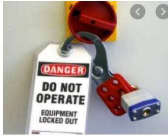
Fig.4. Electrical Lock-out system
