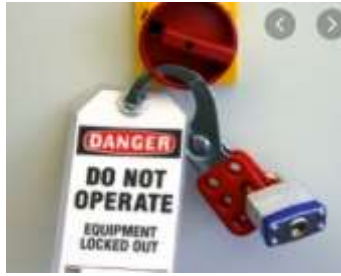
Fig.4. Electrical Lock-out system
