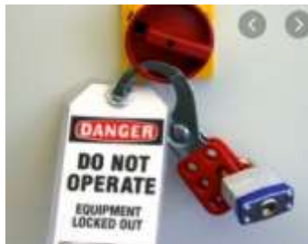
Fig.4. Electrical Lock-out system
