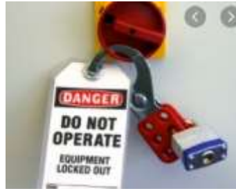
Fig.4. Electrical Lock-out system
